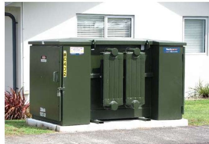
Figure 9.39: Ground-mounted distribution transformer
