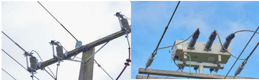
Figure 9.16: Crossarm assembly with drop-down fuses (left) and double crossarm arrangement (right)
