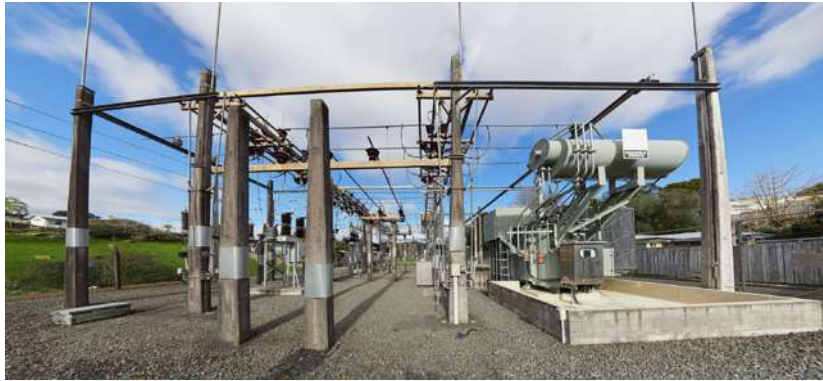
Figure 9.21: Tikipunga zone substation outdoor switchyard
