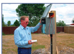
Northpower inspector, Leo Hay testing a temporary supply.
