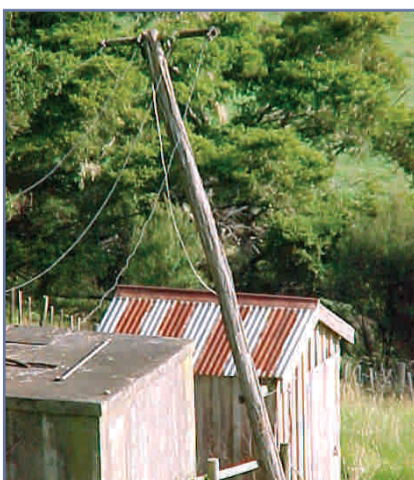
Serviceline pole requiring replacement.
